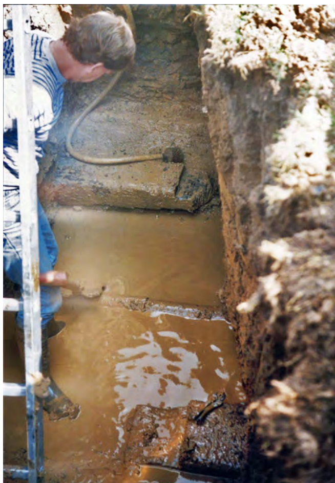
The two longitudinal sleepers with the drain pipe between them are clearly visible in the trench. As the sleepers were 4' 8½" apart (standard gauge) this confirms, beyond reasonable doubt, that Rammell's tunnel had been found
